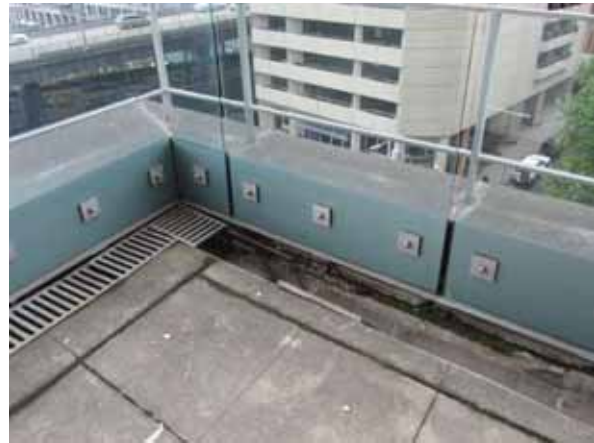
MODERN GLASS BALUSTRADE, DEGRADED CONCRETE DRAINAGE
