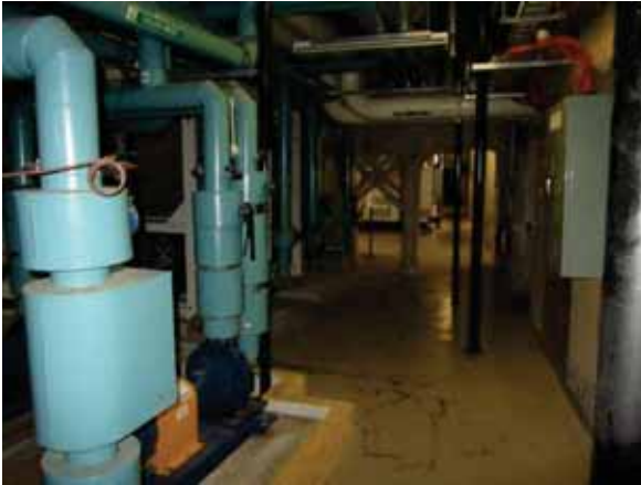
MAINS SECONDARY WATER SUPPLY PLANT
